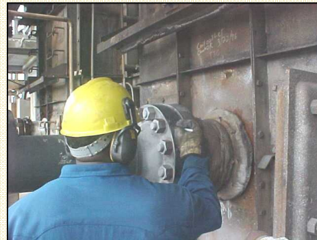
"Hot bolting" (replacing bolts on a flange when the line is still in service)
