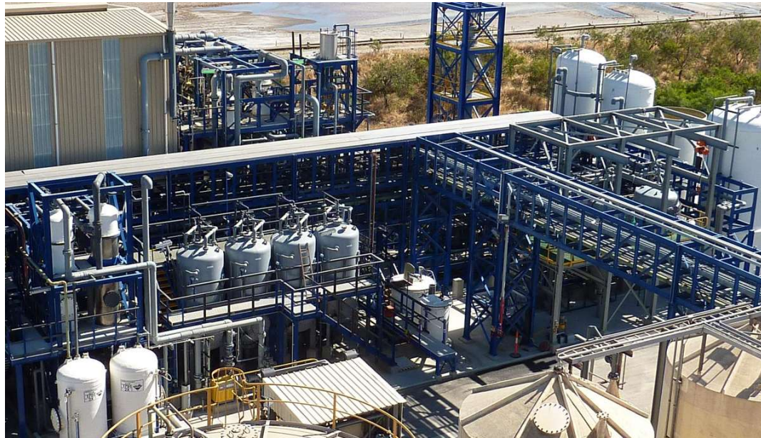
150TPD SKID MOUNTED PLANT
