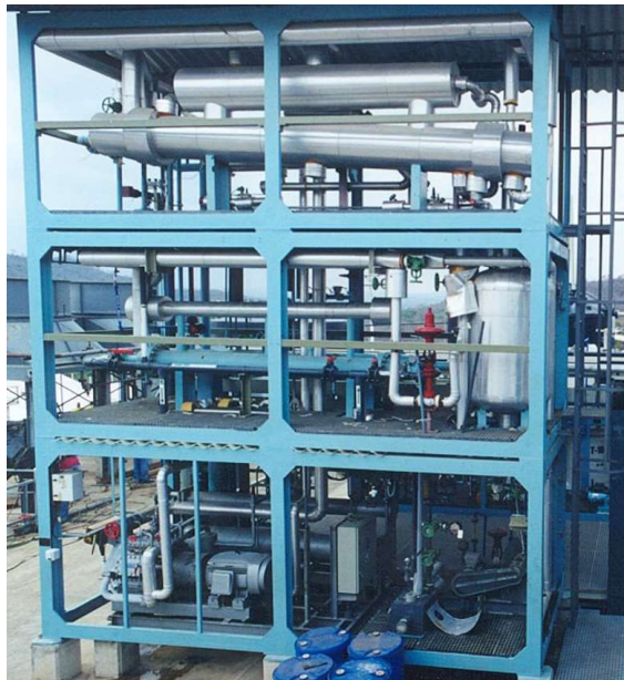
12 TPD CL2 LIQUEFACTION SKID
